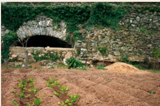
The culvert collects the water to supply Font del Portal and the village water tank
